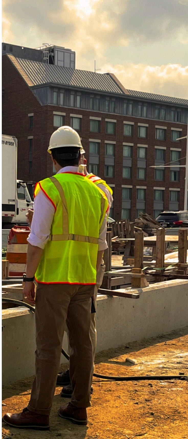
In July 2024, the ISAU team made a site visit to inspect the construction of the William Felton ‘Bill’ Russell Bridge in Boston, which connects Charlestown to the West End and North End.
